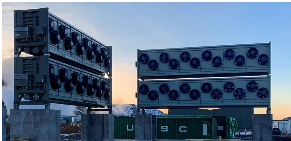
Figure 19: Climeworks CO 2 LT-DAC modular units installed around Carbfix central storage facility at Orca plant. (158)
