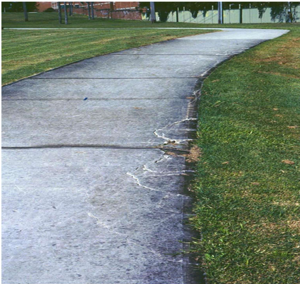
Figure 7. The transverse cracking and settlement near joints in the footpath of Randwick, NSW. (Sagoe-Crentsil, 2002)
