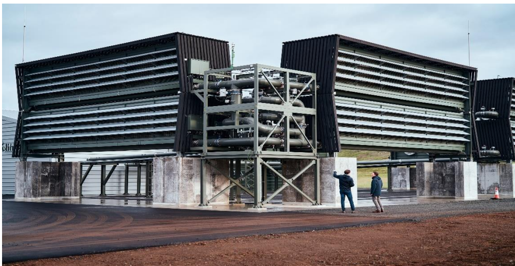
Figure 11: Carbon capture & storage plant located in Iceland
