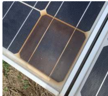
Figure 2.20: Image of an actual hot-spot from the Pedrosa (AL) solar plant.
